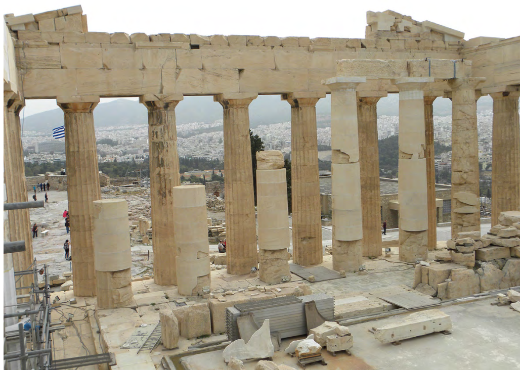
Figure 35.8 Implementation of Korres-Bouras' proposal for partial restoration of Pronaos 2004, view from northwest. Source: L. Lambrinou.
