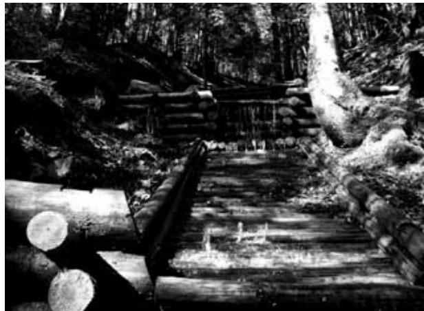
Fig. 3.4 River restoration work using belts, stones, wood, and plant material for slope and river bed protection (Pavlidis, 2012).
