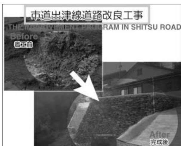
Fig. 6 A stone wall before and after maintenance and recover (photo by the Office)
